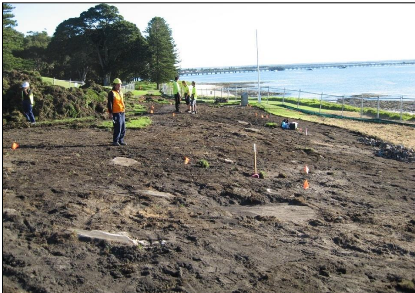
Figure 32. Monitoring of pathway installation near the main flagpole east of the stream.
