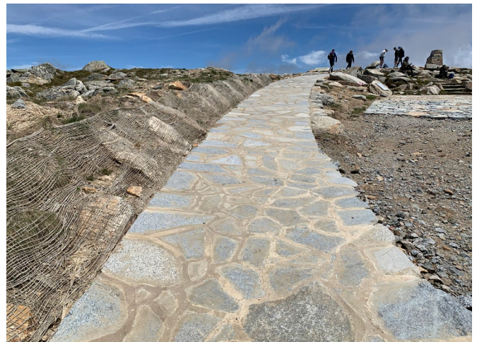
The new low mobility access ramp leading to the top of Mt Kosciuszko. Photo: J Crawford / DCCEEW
