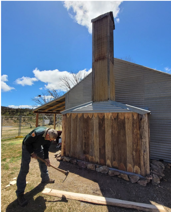
NPWS builder adzing chimney slabs on the recently rebuilt Bradley & O'Brien's Hut. Photo: M Bowden / DCCEEW
