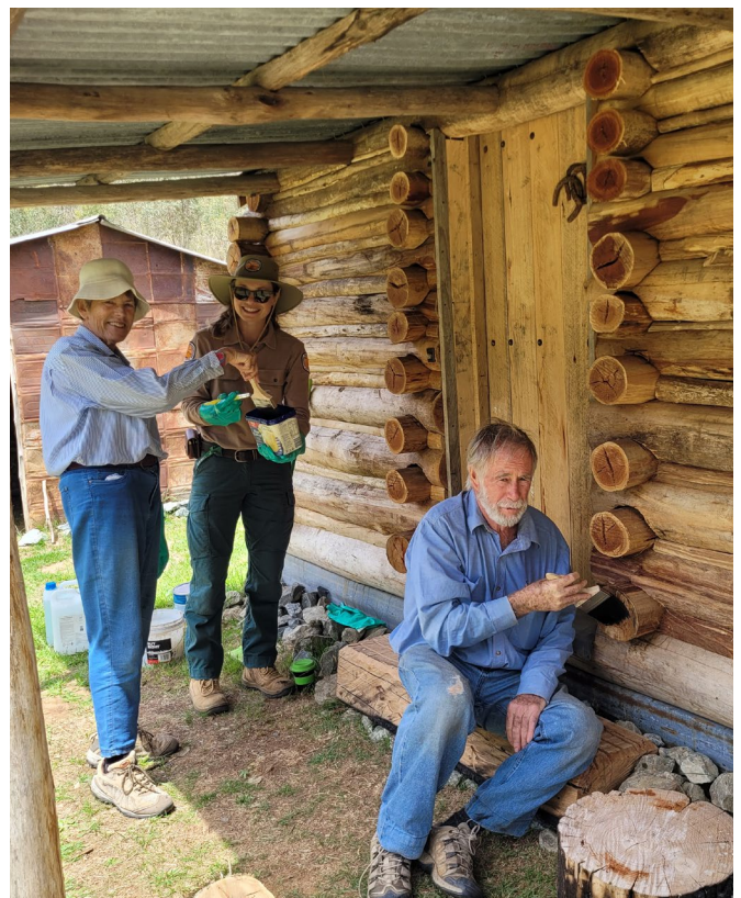
NPWS Ranger & KHA volunteers applying fire retardant to Vickery's Hut #2. Photo: G. Johnston / DCCEEW
