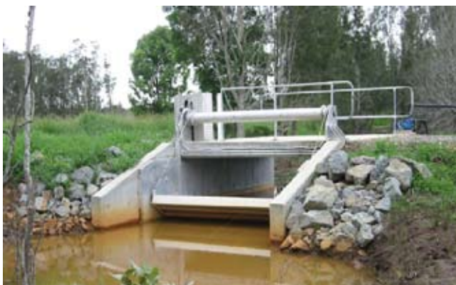
Plate 18. Water retention gate at Partridge Creek on the Hastings River floodplain
