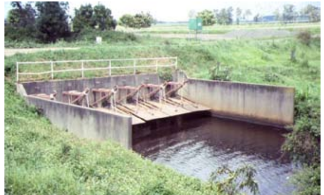
Plate 15. Floodgate lifting devices From top: a) Lifting devices on headworks on the Belmore River on the Macleay
