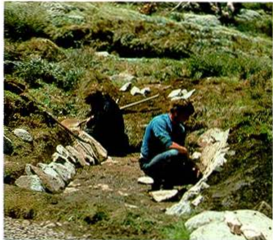
Stone drains and contour banks were constructed by hand to control runoff - this was time consuming and back breaking work.
