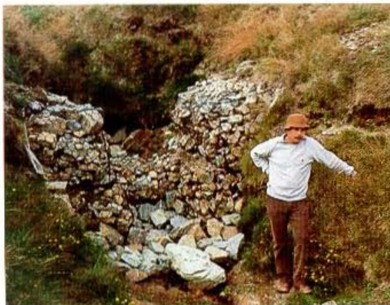
One way to stabilise large and badly eroded gullies is to use rock filled baskets called gabions. These are placed at the head and along the sides of the gully to prevent mass movement of soil.
