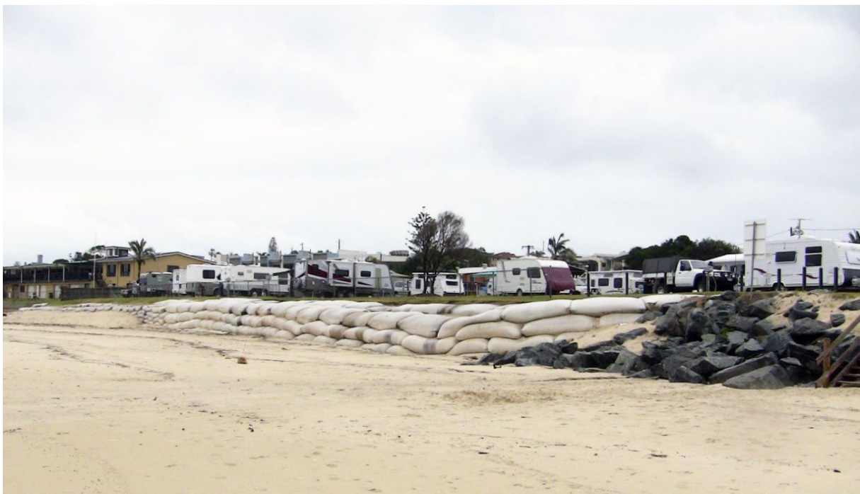
Coastal erosion management, Kingscliff Beach. Photo: P Davies/DCCEEW
