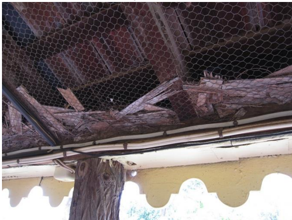
Underside of verandah shingles and chicken wire.
