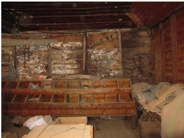
North wall of Store, deteriorated under central valley.
