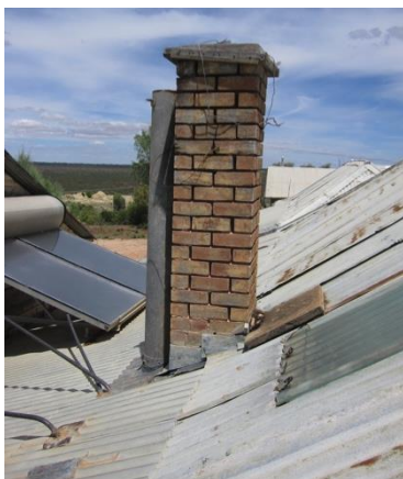
Kitchen chimney with capping slab on roof to right. Corrugated glass skylight to right or photo.
