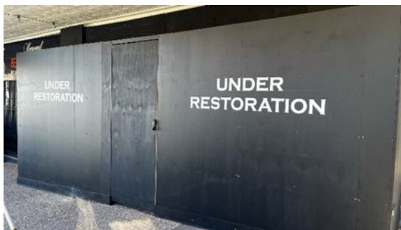
Image: Restoration hoarding installed to the front of the Paragon Café (Source: Heritage NSW)
