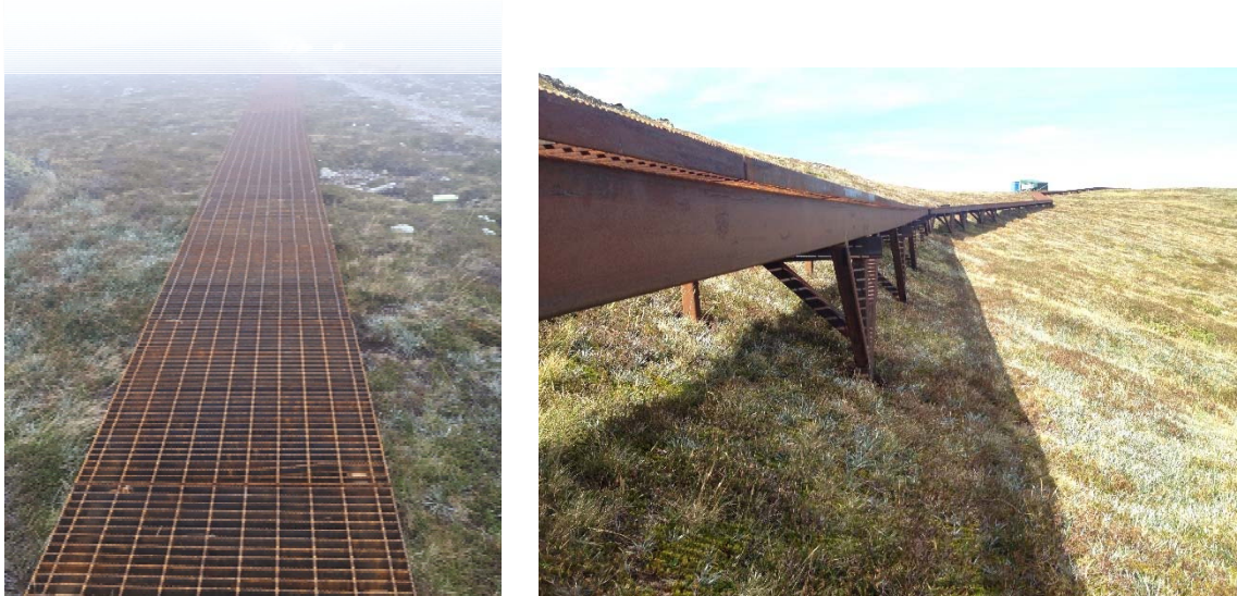
Figure 1: examples of raised steel mesh walkway constructed at Mt Lee, Main Range, Kosciuszko NP
