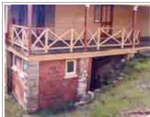
PHOTO 5.2-8 DETAIL OF EDGE TREATMENT BETWEEN BUILDING AND COURTYARD AREAS WHICH ARE DIFFICULT TO MAINTAIN TBLD P/L
