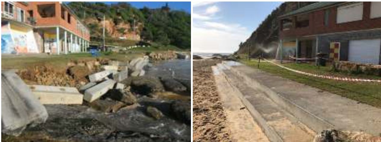
Plate 7: Left: Nambucca Main Beach Surf Club access stairs damaged by storm events; Right: Main Beach Surf Club after replacement of access stairs
