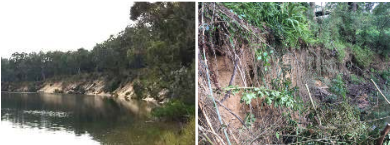
Plate 11: Left: Unstable unconsolidated sand banks in Warrell Creek (July 2018); Right: Severe bank instability and undercutting on the South Arm, upstream of Bowraville (July 2018)
