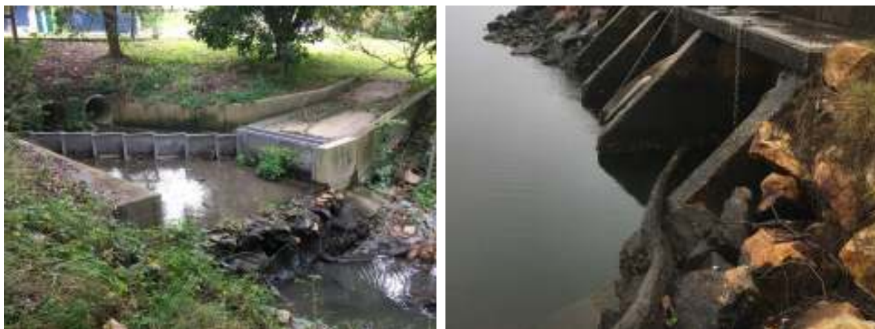
Figure 7: Left: Gross Pollutant Trap at Bellwood Park; Right: damaged floodgate at East Street, Macksville (July 2018)
