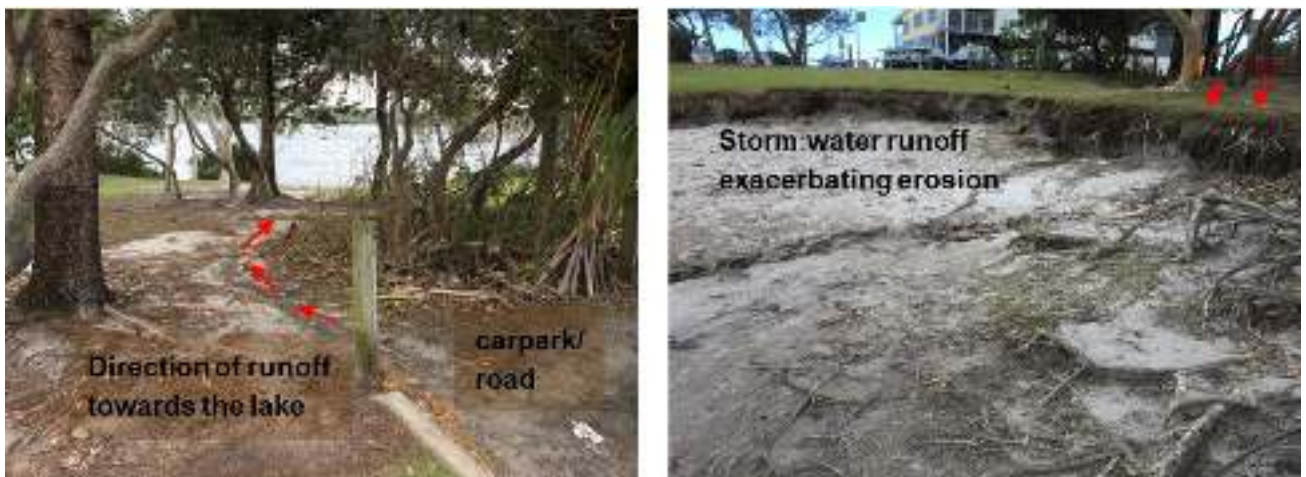
Plate 7: Foreshore erosion at the lake
